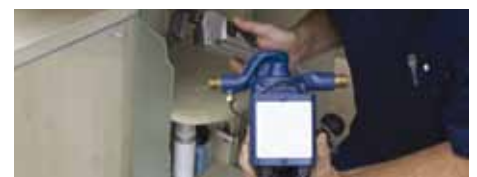
Water recirculation devices are usually located under kitchen or bathroom sinks
