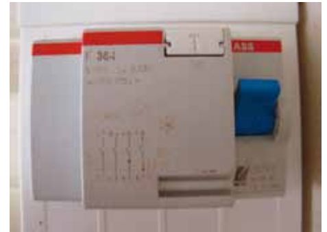
Check your meter box or switchboard to see if you have an electrical safety switch
