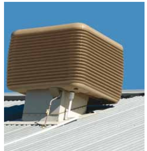
The main unit of an evaporative air-conditioner is usually located on the roof
