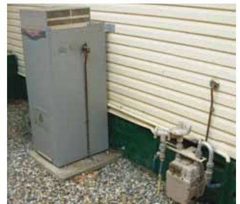
An example of a gas storage hot water system
