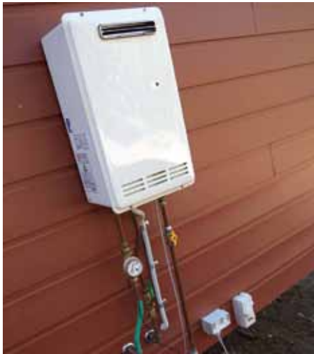
An instantaneous gas hot water system
